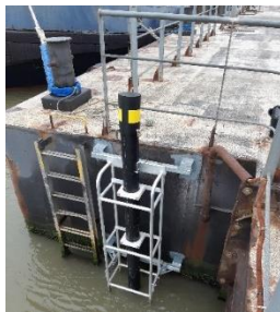
Figure 1 : Station SYVEL de Montoir-de-Bretagne
